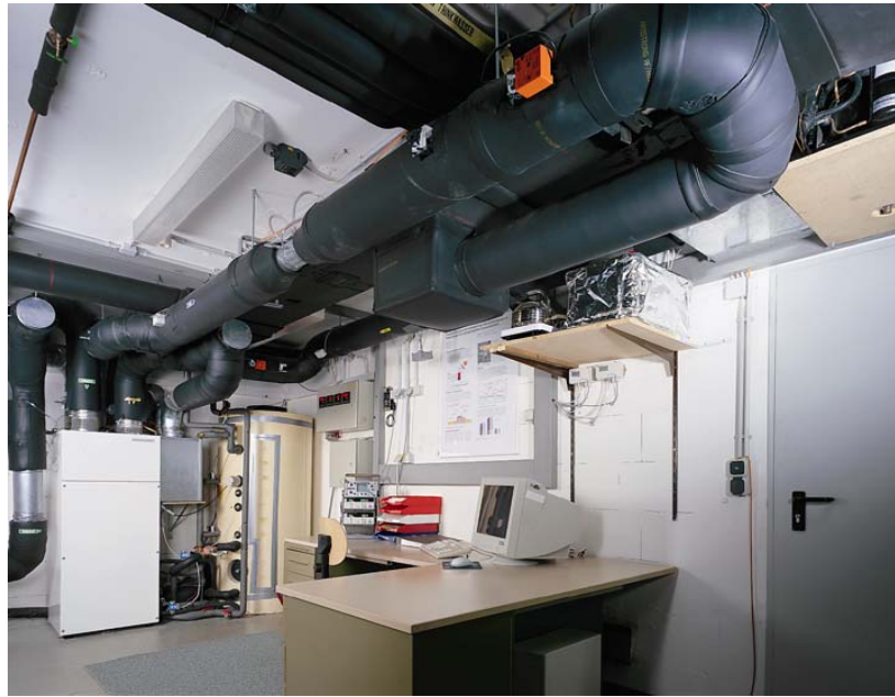
Fig. 3. Test facility in the Freiburg Solar House, with room for two compact ventilation devices with an integrated exhaust air heat pump
