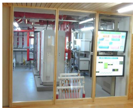
Visible GSHP machine room and displays
