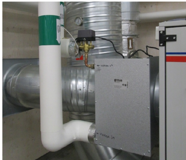
Figure 9: The preheater installed on the existing dehumidifier in ice rink A.
