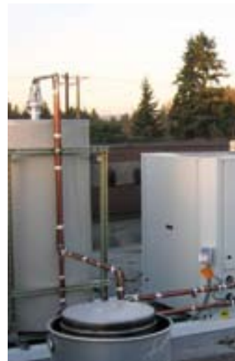
Picture: Joint Carrier / US DOE CO 2 heat pump water heater prototype installed in Oregon
