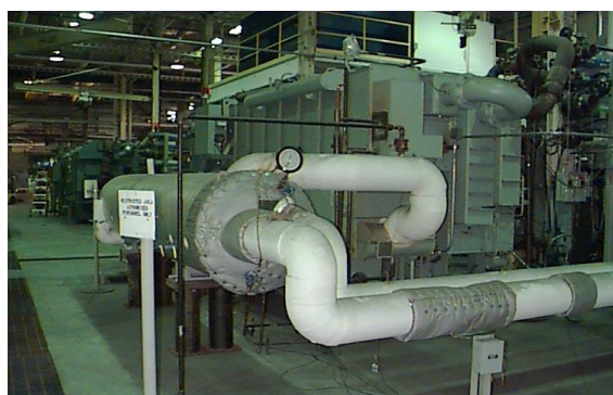
Figure 4. Triple-Effect, Exhaust-Heat-Fired Absorption Chiller Tested at York International, York, Pennsylvania.
