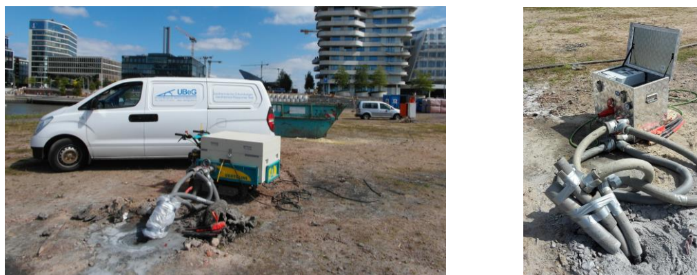
Fig. 8. Typical TRT-setup at BHE on a site under development, in summer 2016 (left) and very mobile TRT on the same site in Northern Germany (right), photos Kahl/UBeG
