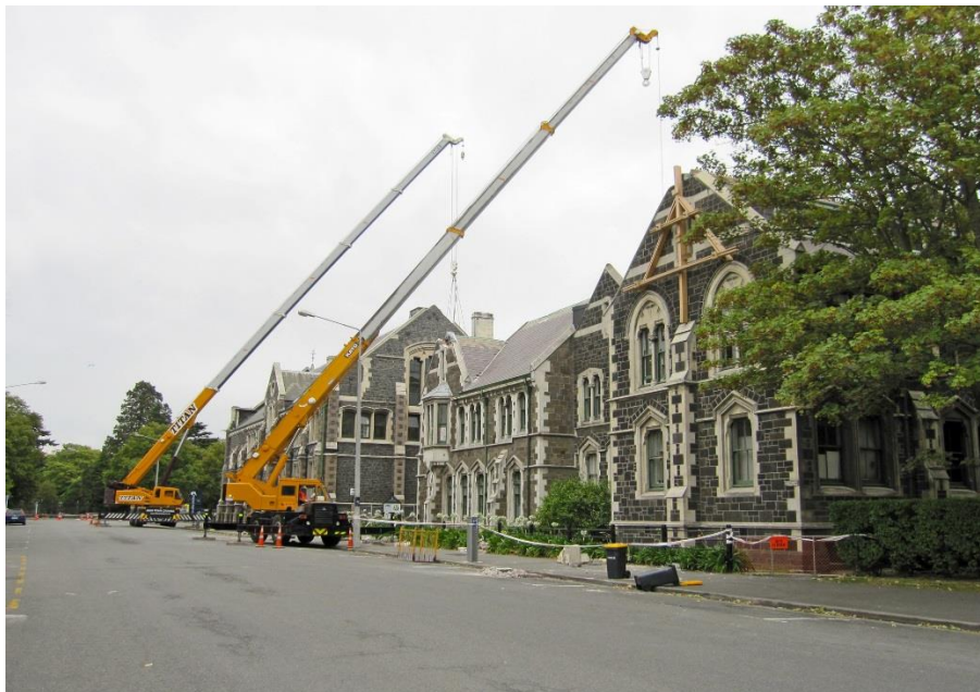
Fig. 3. Photograph of cranes removing masonry from the Art Centre March 2011 (Margaret Low, GNS Science)
