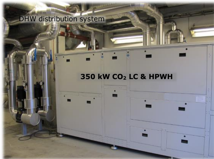
Fig. 9. The CO 2 liquid chiller (LC) and HPWH installation at UNN, Tromsø (Photo: Kuldteknisk AS, Norway).
