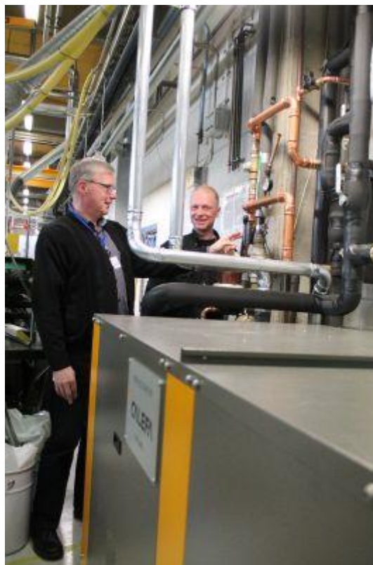
Figure 5. Plastep Heat pump system in operation
