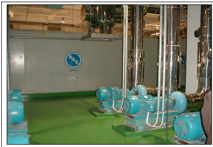
Figure 4. Ice Thermal Storage units installed in the basement
