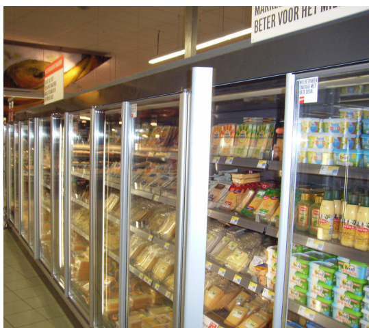
Figure 1. Refrigeration accounts for close to 50 % of the electrical energy consumption of a supermarket.
