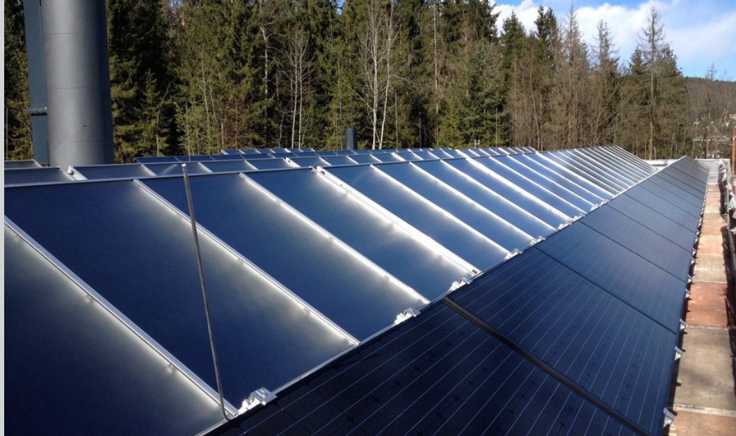
Fig 1: Solar thermal system at the biomass heating plant Krumpendorf [Regionalwärme, 2017].
