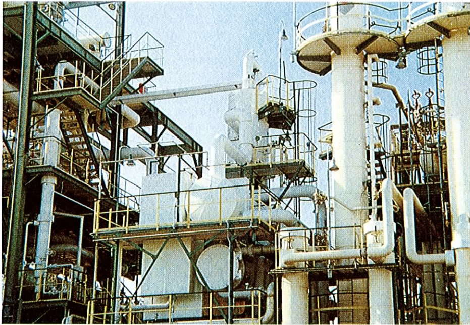
2.35 MW Type II Absorption Heat Pump in a Butadien Rubber Plant in Japan. This Waste Vapor source heat pump supplies regenerated steam to the distillation tower (see also page 9) Photograph JRAIA
