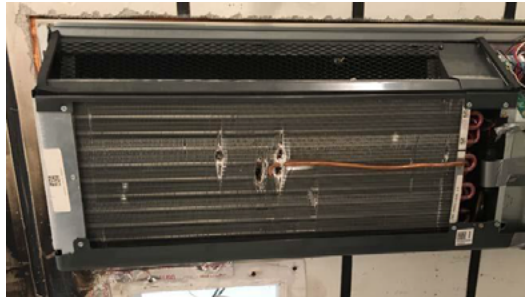
Fig. 2. PTAC discharge tube location [2]
