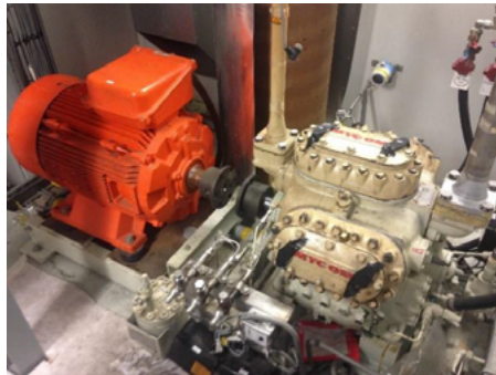
Figure 3: HP Mayekawa piston compressor
