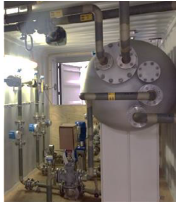
Fig. 5. Internals of test rig showing the buffer vessel and ancillary components
