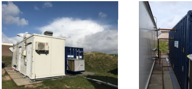
Fig. 1. Containers which house the heat pump (white container) and test infrastructure (blue container) and associated connections
