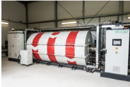
Figure 9: RHP-K7, field installation
