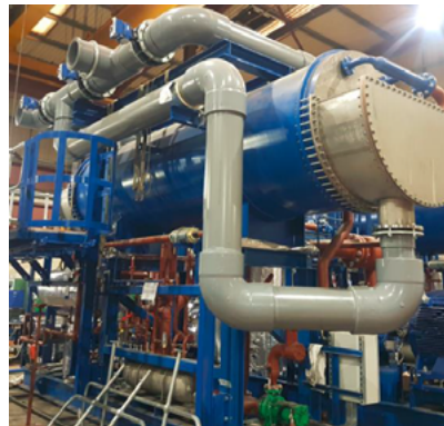
Fig. 6. Flow Reversal Pipework On the Side of the Spray Chiller Evaporator
