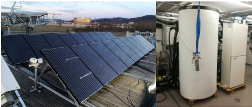
Fig. 3: Investigated single source SHP system with an array of PVT collectors in two rows totaling 20 collectors installed on top of the system test stand at Fraunhofer ISE (left). The photo on the right shows the installed combi storage and the heat pump including a hydraulic unit. The power inverter is installed as well (not shown in the photo).
