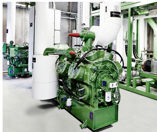
Installation of a hybrid absorption/compression heat pump using a mixture of water and ammonia at Arla, Denmark
