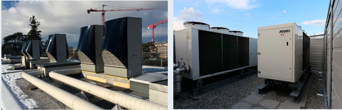
Figure 2: Two rooftop projects with air-to-water heat pumps realized in Geneva. Right: industrial heat pumps with over 80dB(a) at emission with surrounding noise-reduction walls (Source: SIG/ CSD Ingénieurs SA)
