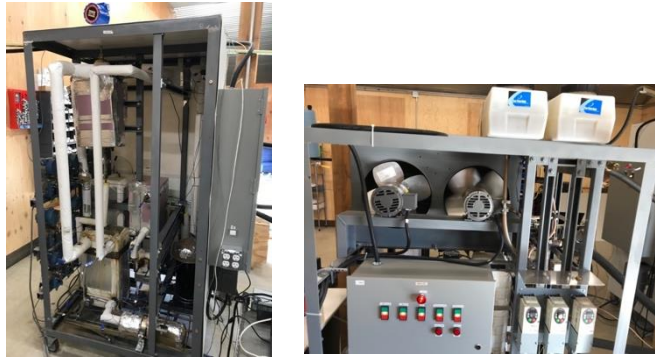
Figure 8 Photos of the Actual HTHP Prototype System
