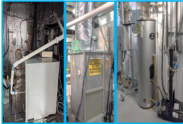
Figure 2: The “Hybrid” GAHP-EAC unit. (Left) The outdoor unit in the environmental chamber; (Middle) The AHU unit system; (Right) The 80-gallon storage water heater.
