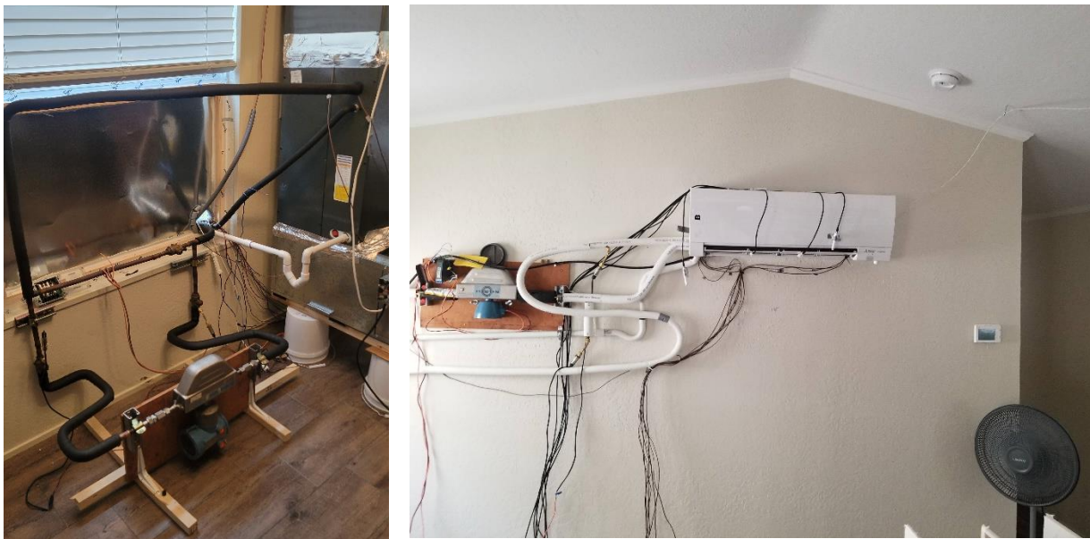
Fig. 10. Ducted (left) and Ductless (right) Indoor Units, Showing Refrigerant Mass-flow Sensors.
