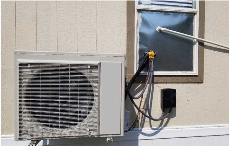
Fig. 8. Typical Ductless Outdoor Unit Installation, Showing Steel Window Replacement.
