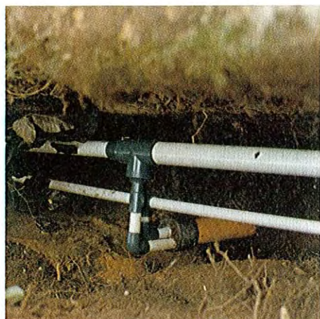
Photo 2 Connection of Heat Exchanger Tube to Flow and Return Manifolds
