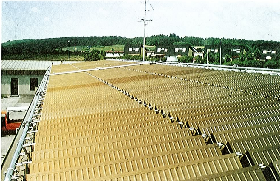
Fig. 4 View of the installed roof absorber with a surface of 500 m 2 in Engen
