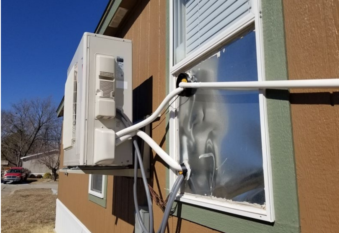
Steel window panels increased load
