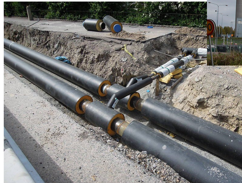
Typical district heating piping in street in Sweden
