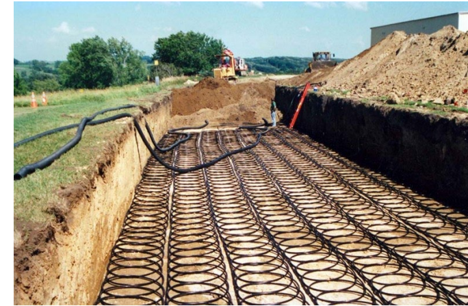
Ground Source Heat Pump 3
