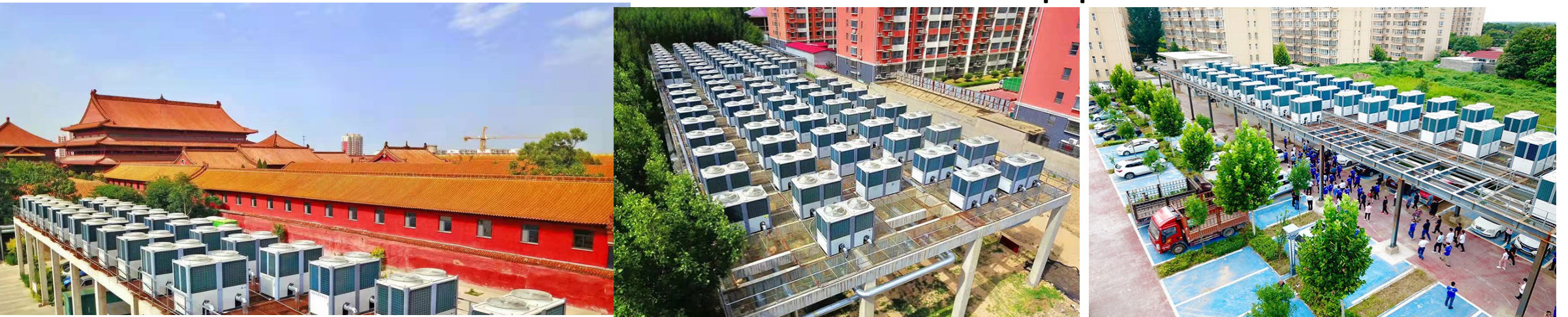
Fig.3: ASHP installation sites
