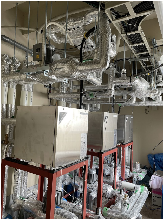
GSHP units in 1st floor
