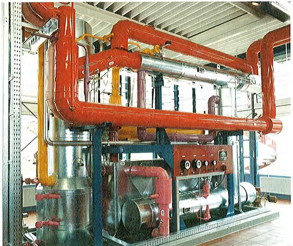
Fig.1: Single-stage gas-fired air-source absorption heat pump of the TWS
