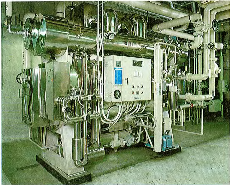
Fig. 1 Absorption heat pump (Tokyo Gas, Shinjuku Bldg.)
