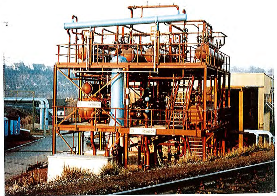
Fig. 3 AHP demonstration project "Fernwärmeschiene Saar", F.R. Germany (Borsig GmbH).
