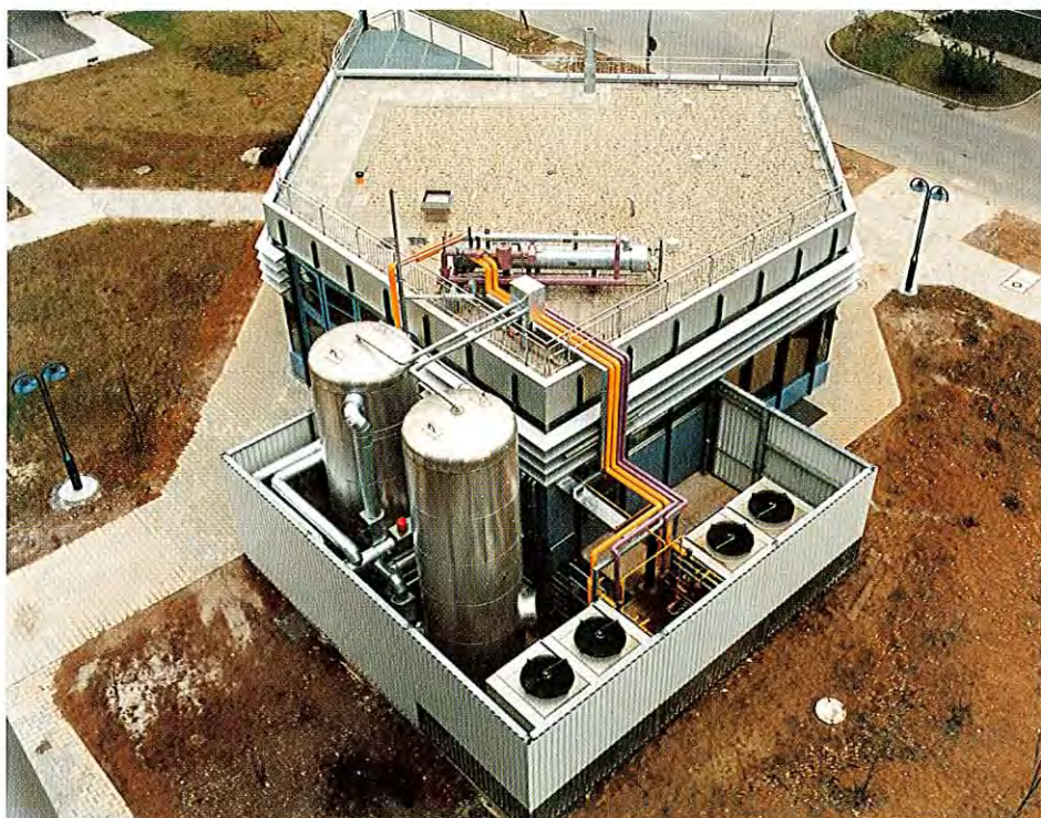
TWS-Absorption heat pump in Stuttgart; Engine house with air evaporators and hydraulic buffer storages (see page 7).
