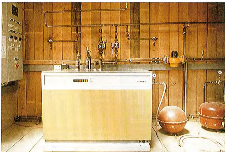
Fig 3. Siemens heat pump used at Schwalbach GCHP Research Station
