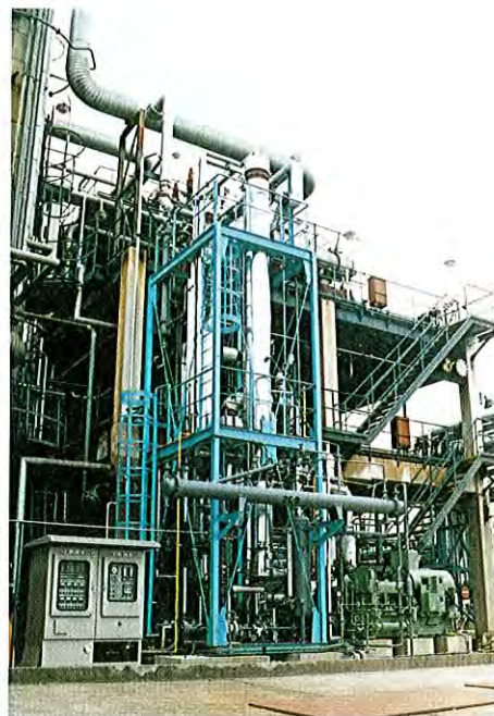
Fig. 1 Pilot plant of a high-efficiency and high-compression-ratio heat pump system with water as working fluid
