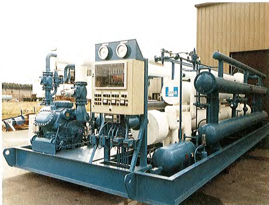
Figure 2. Heat Pump Used for Live Lobster Storage (Before Installation)
