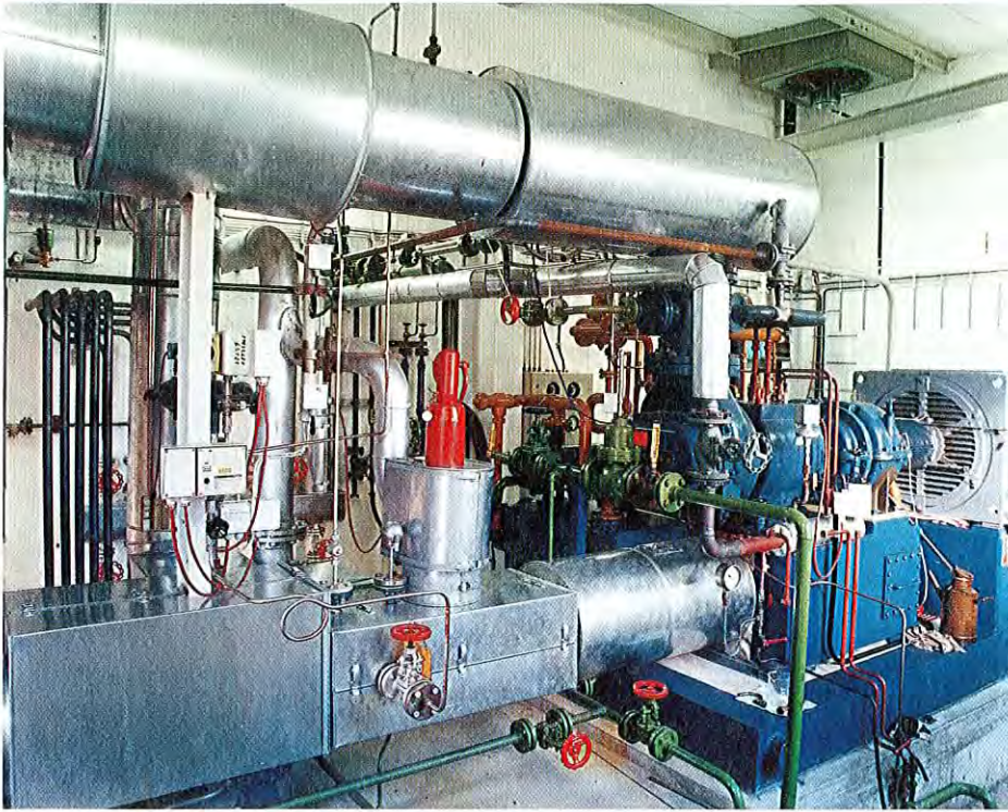
Figure 1. Pilot plant for steam compression
