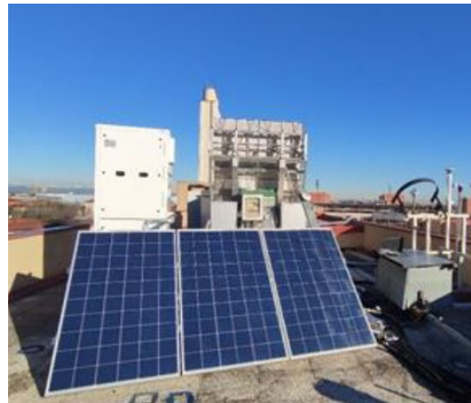
Figure 3-14 - Solar assisted heat pump prototype working with CO 2 installed at the Solar Energy Conversion Laboratory (Department of Industrial Engineering, University of Padova).
