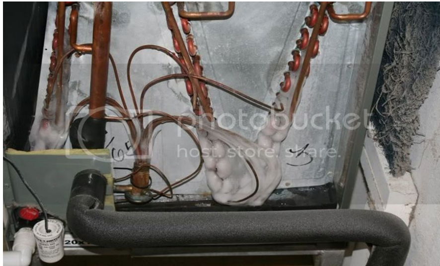
Figure 3-3: Bad distribution example.
