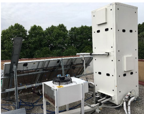
Figure 3-22a. Heat pump prototype installed at the Solar Energy Conversion Laboratory (University of Padova).
