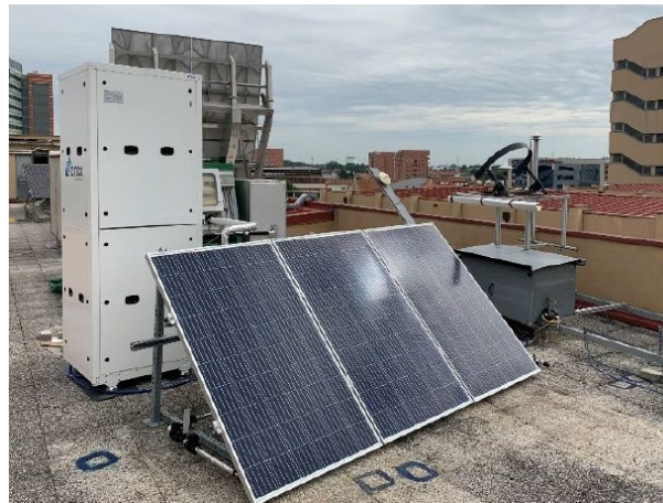
Figure 3-6: Solar-assisted heat pump prototype was installed at the Solar Energy Conversion Laboratory (Department of Industrial Engineering, University of Padova).
