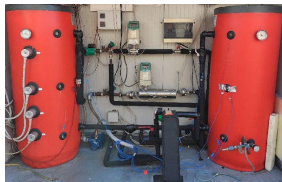
b. Picture of water tanks, brazed plate heat exchanger and flow meters installed in the water loop.
