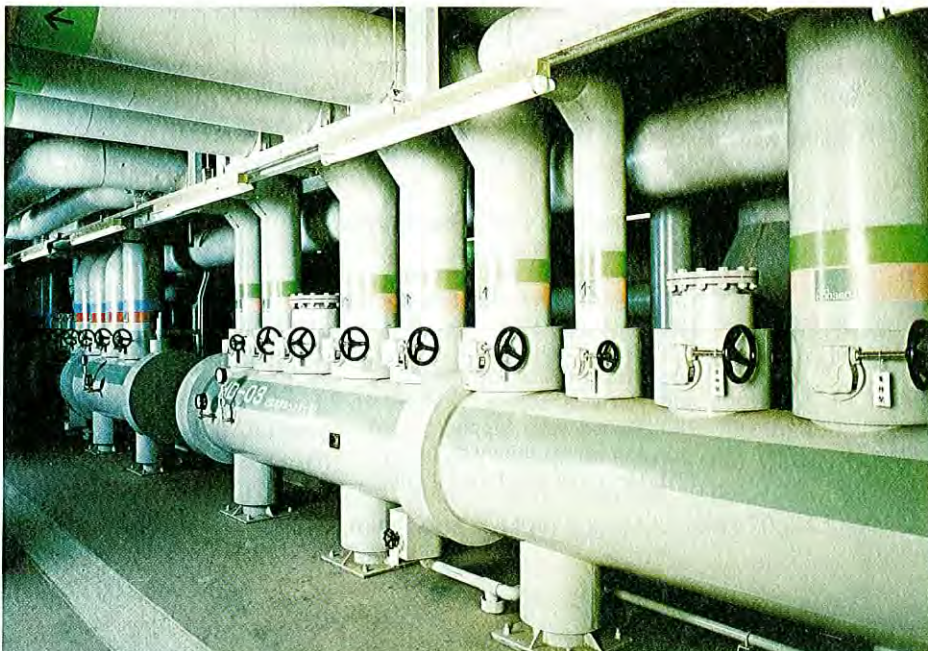
Figure 4. Chilled/hot water secondary supply header
