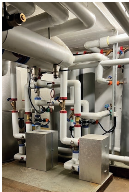
Figure 2: Heat pump installation in the cellar of the building (in the place of the old oil-burner) St. Julien, Geneva, Switzerland.
