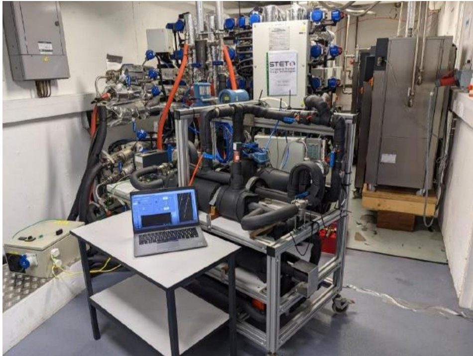
Figure 5. Image of the proof-of-concept resorption experimental rig in front of the ThermExS test facility
