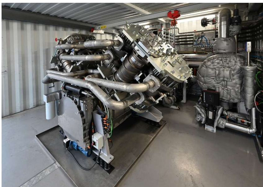
Figure 2. HoegTemp HTHP with steam generator, as installed at GE Healthcare, Lindesnes, Norway
