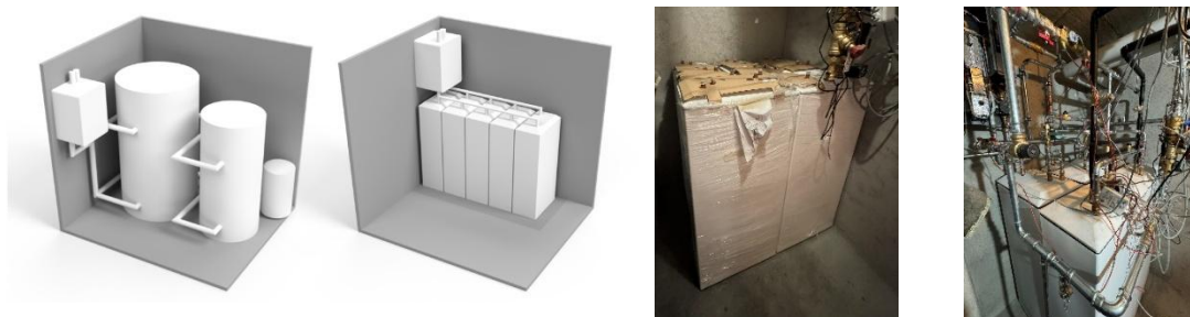
Figure 9. Comparison of installation space (left) and Compact Cell installation in Pany (right)
