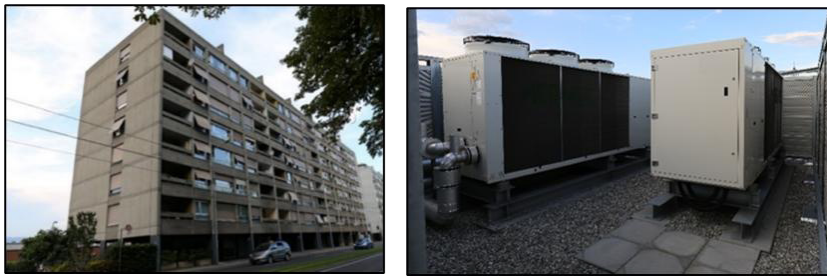
Figure 1. Non-retrofitted MFB (left) equipped with two air-source HP on the roof (right).
