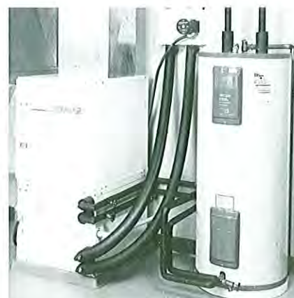
Front Cover: In the US, utilities, government agencies, research institutions, and public interest groups are working together to stimulate the market for ground-source heat pump installations such as this one. Further details are given in the article on page 20.
