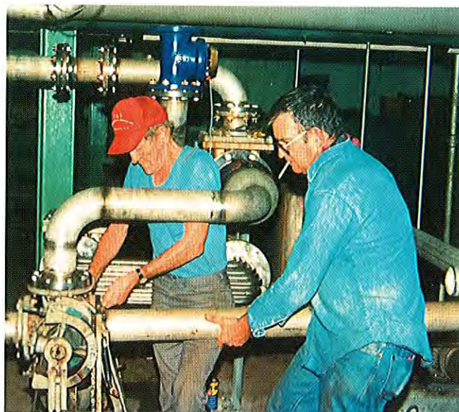
Photo 2: New equipment at the A&E's thread plant including a trash pump (right) and a reversing valve (centre).
