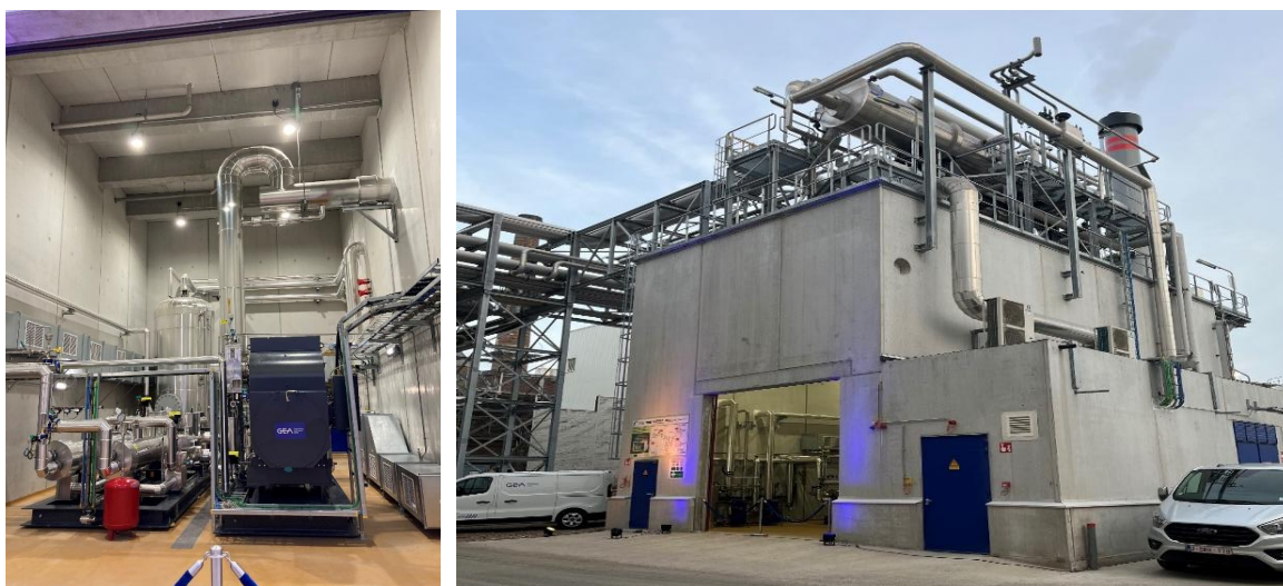
Figure 3. Pictures of the GEA heat pump installed on-site in Tienen.
