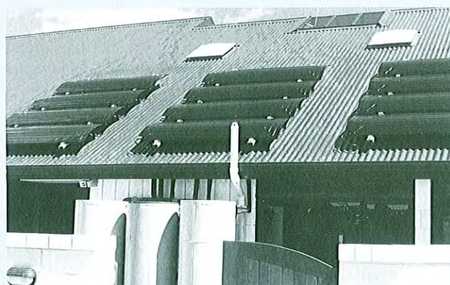
Photo 2: Hot water from thin air: rooftop collectors supply free heat to heat pump water heaters.
