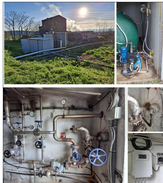
Figure 4. Geothermal data logging facility at the GEOSYN geothermal well.
