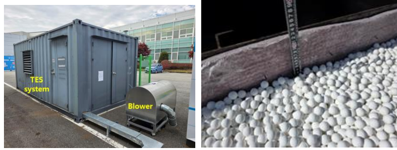
Figure 2. Photo of TES system
