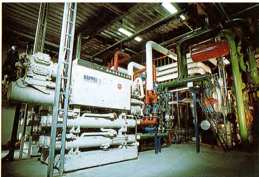
Photograph 1: Heat Pump Unit with Three Refrigerant Circuits.
