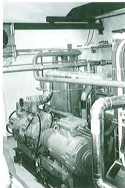
In the services: This ammonia heat pump serves a military base in Norway (source: SINTEF).
