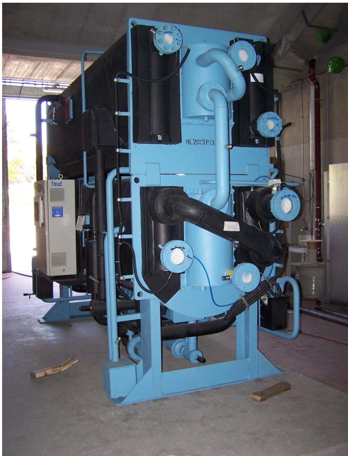
PHOTO 2: TWIN Design Hot water driven Absorption Heat Pump at STADTWERKE, GERMANY.
