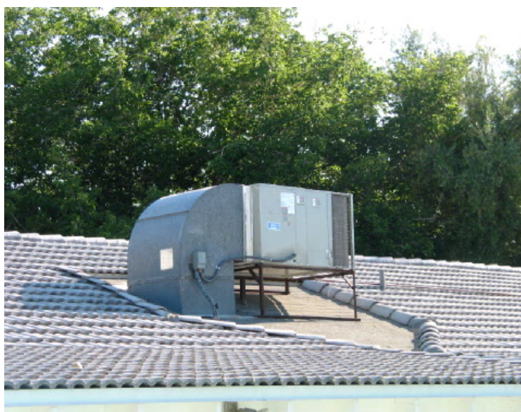
Figure 6 Rooftop Single-Package Heat Pump Installation in Las Vegas
