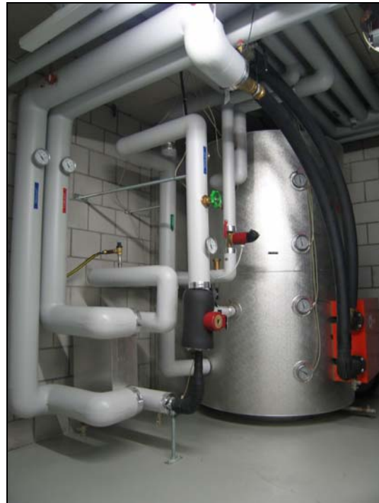
Figure 3: hot water tank: external heat exchanger (at left) and internal heat exchanger (at right), that is only mounted provisionally
