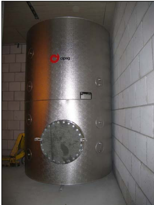
Figure 2: hot water tank: the manhole cover gives an inkling of the size of the heat exchanger that was mounted later
