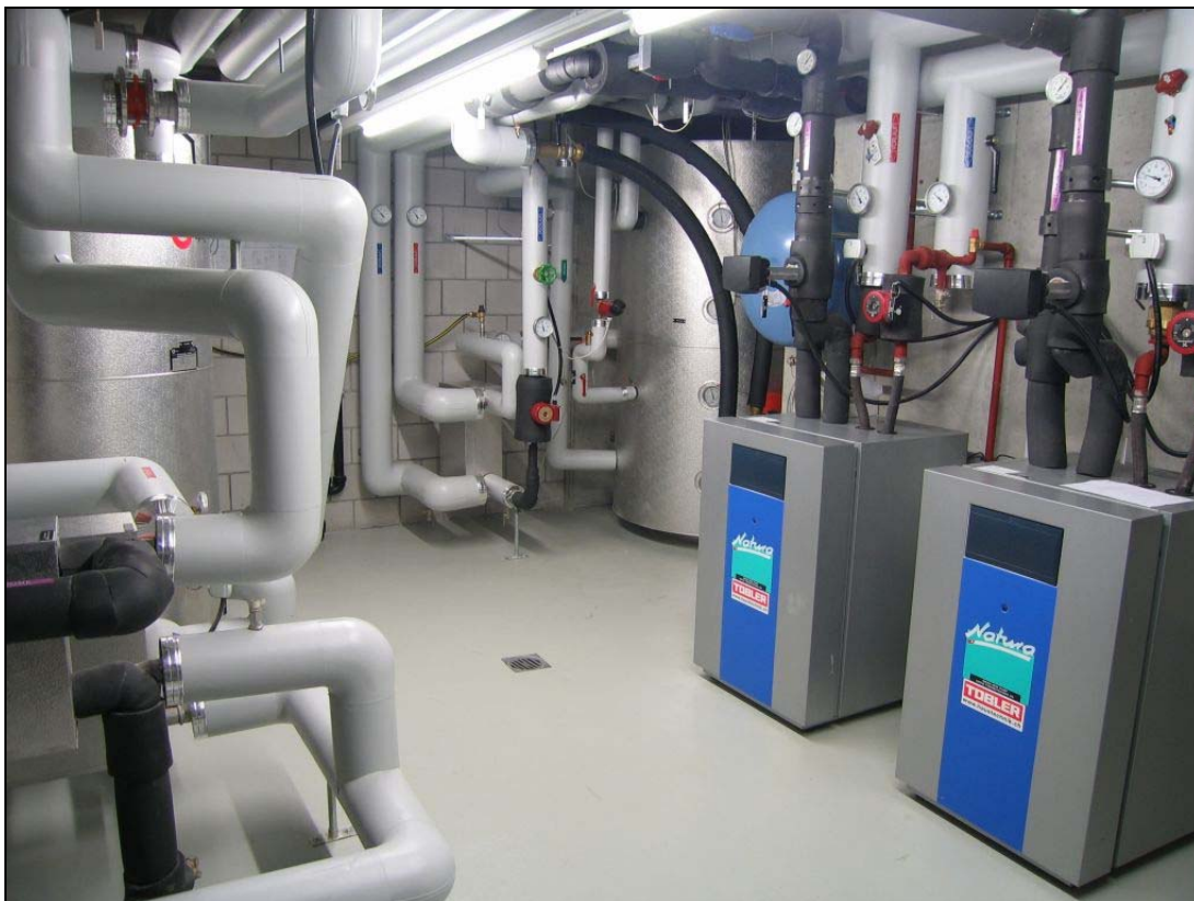
Figure 1: central heating room: heating tank (at left), hot water tank (at back) manufactured by CIPAG, two heat pumps (at right) manufactured by SATAG
